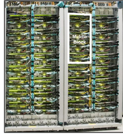
Figure 14: Jupiter Middle blocks housed in racks.
