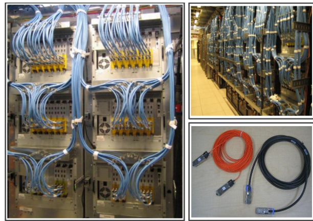
Figure 7: Two Firehose racks (left), each with 3 chassis with bulky CX4 cables from remote racks. The top right figure shows an aisle of cabled racks.
