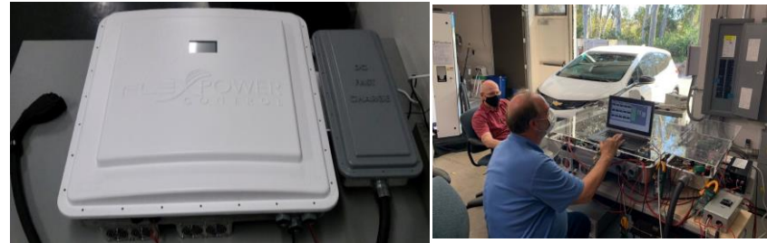
Flex Power SPIN DC V2G + Solar + Storage, tested with Chevy Bolt, August 2021
