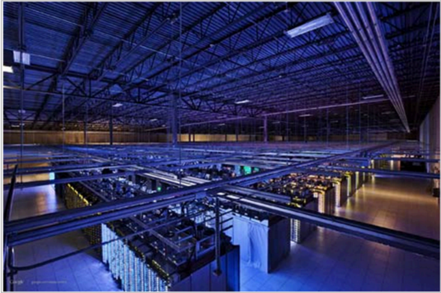
An overhead view of the server infrastructure in Google's data center in Council Bluffs, Iowa, where the company has invested more than $1 billion. (Photo: Connie Zhou for Google)
