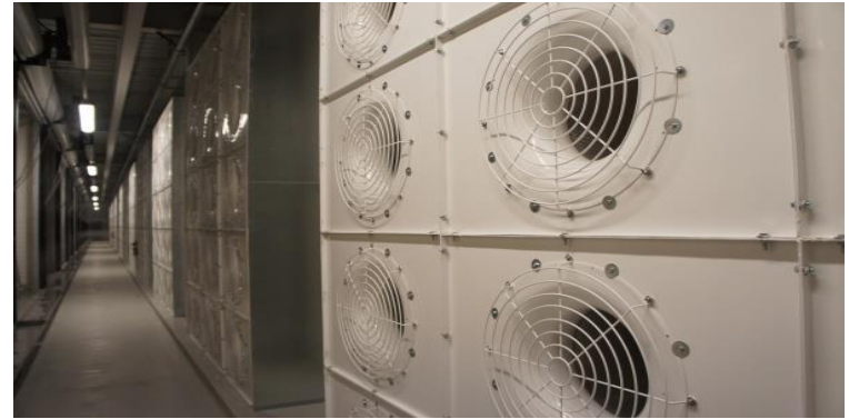
15 motors per server bank
