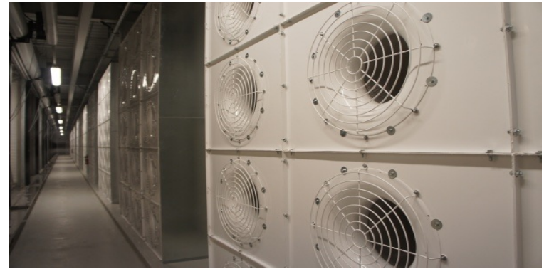
15 motors per server bank
