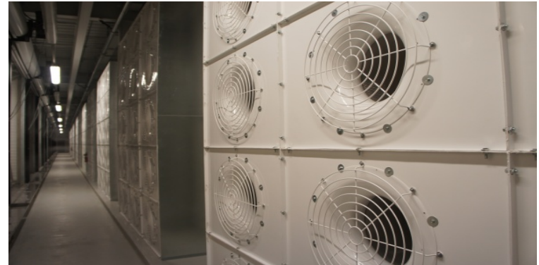
15 motors per server bank
