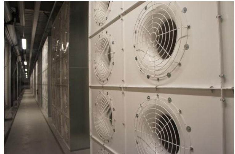
15 motors per server bank
